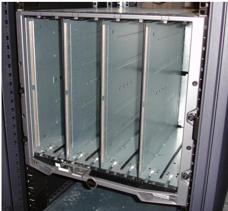
Figure 46. M1000e Mounted in the Rack
