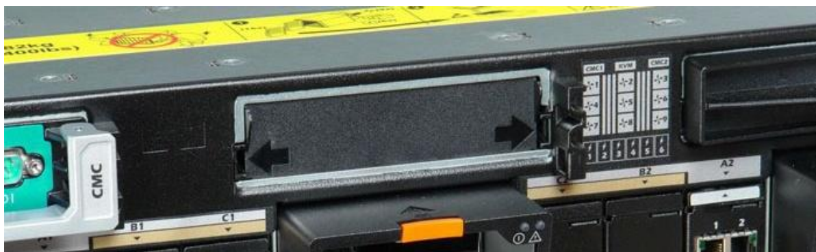
Figure 15. Installed iKVM Blank
