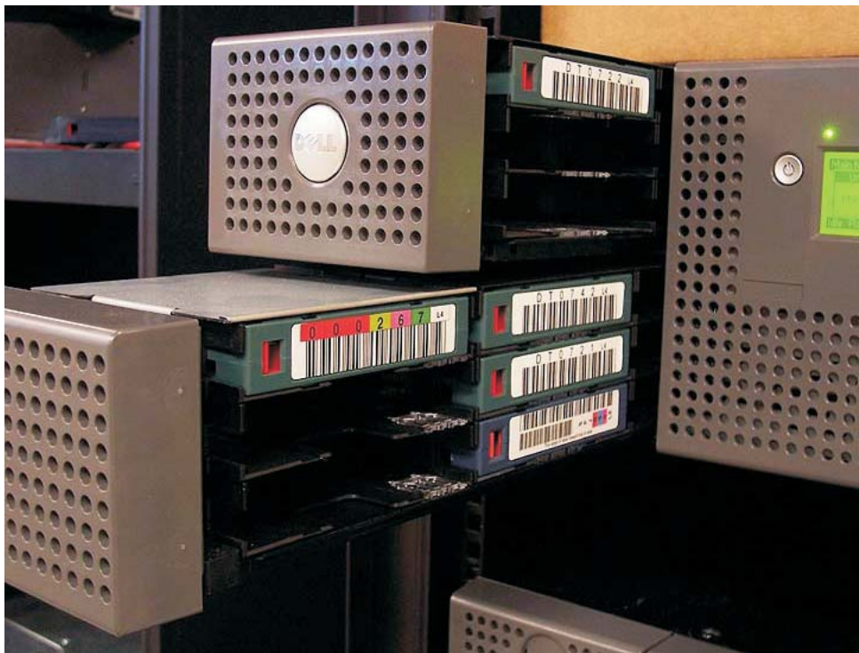
Figure 4-38. 4U library I/O Station in the lower left magazine
