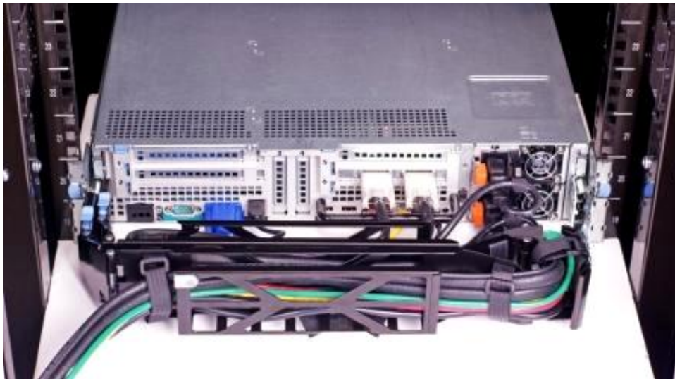
Figure 15. CMA Mounted on the Side Opposite the Power Supplies (Recommended)
